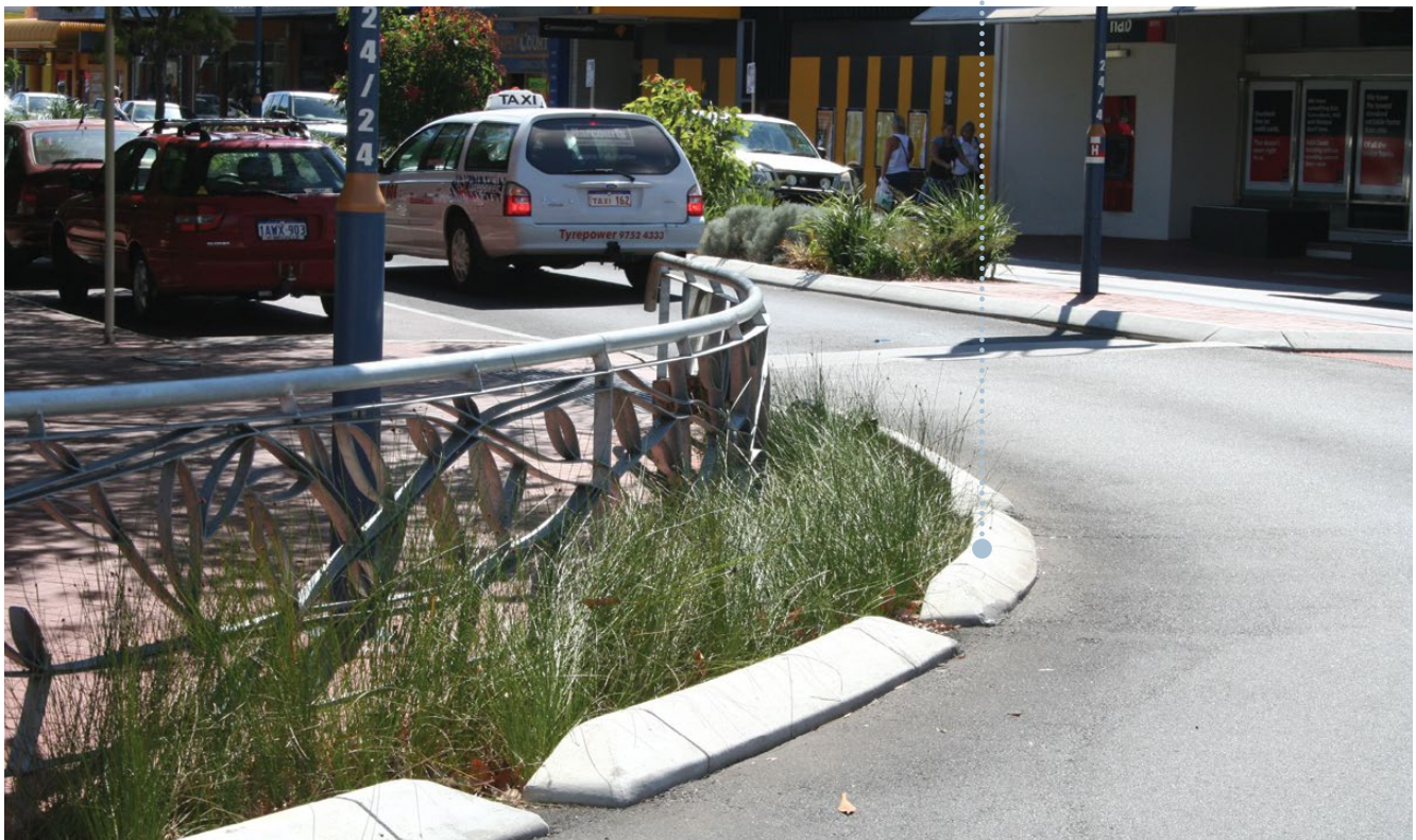
The broken curb and plants together form a stormwater biofiltration solution, retrofitted into a main street shopping area in Busselton, in the south of Western Australia. This is a good example of water sensitive urban design.
